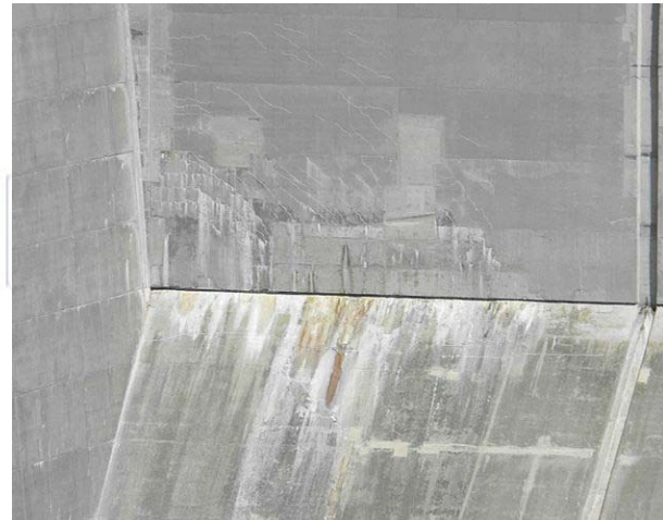
Efflorescence on a concrete face of a dam.
