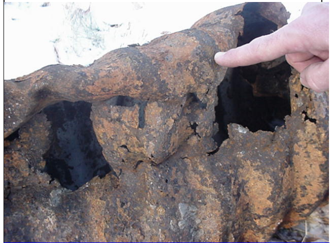
Severely damaged corrugated metal pipe, due to corrosion.
