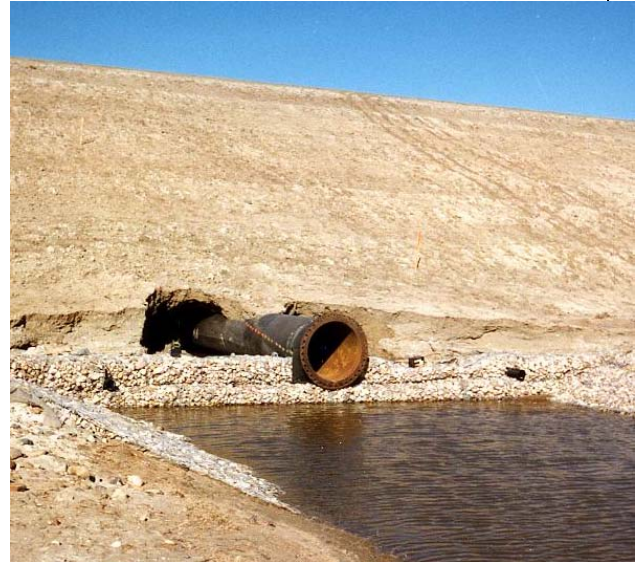
The area around the metal conduit has been eroded away by seepage along the pipe.
