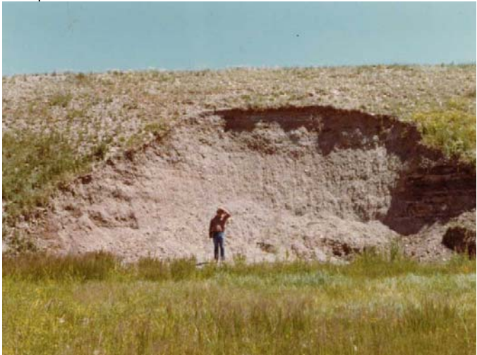
Seepage has severely damaged this embankment.
