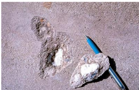
Popouts are caused by the freeze thaw cycle.
