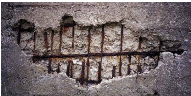
Spalling exposes metal reinforcement to corrosion.
